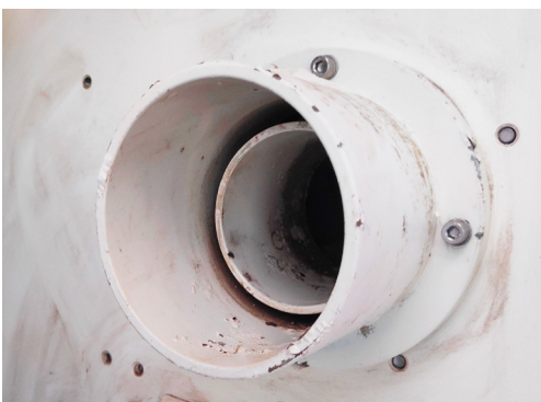
Fig. 37 Ductwork should be foolproof in terms of cracks, leaks or corrosion.
